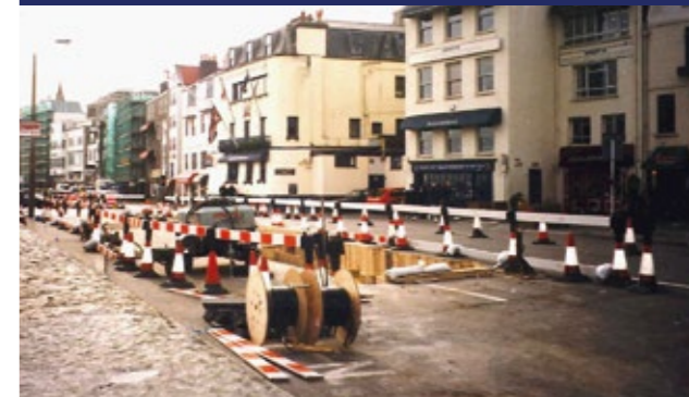
CABLE LINK FROM FRANCE VIA JERSEY BEING INSTALLED AT HAVELET BAY IN 2000
